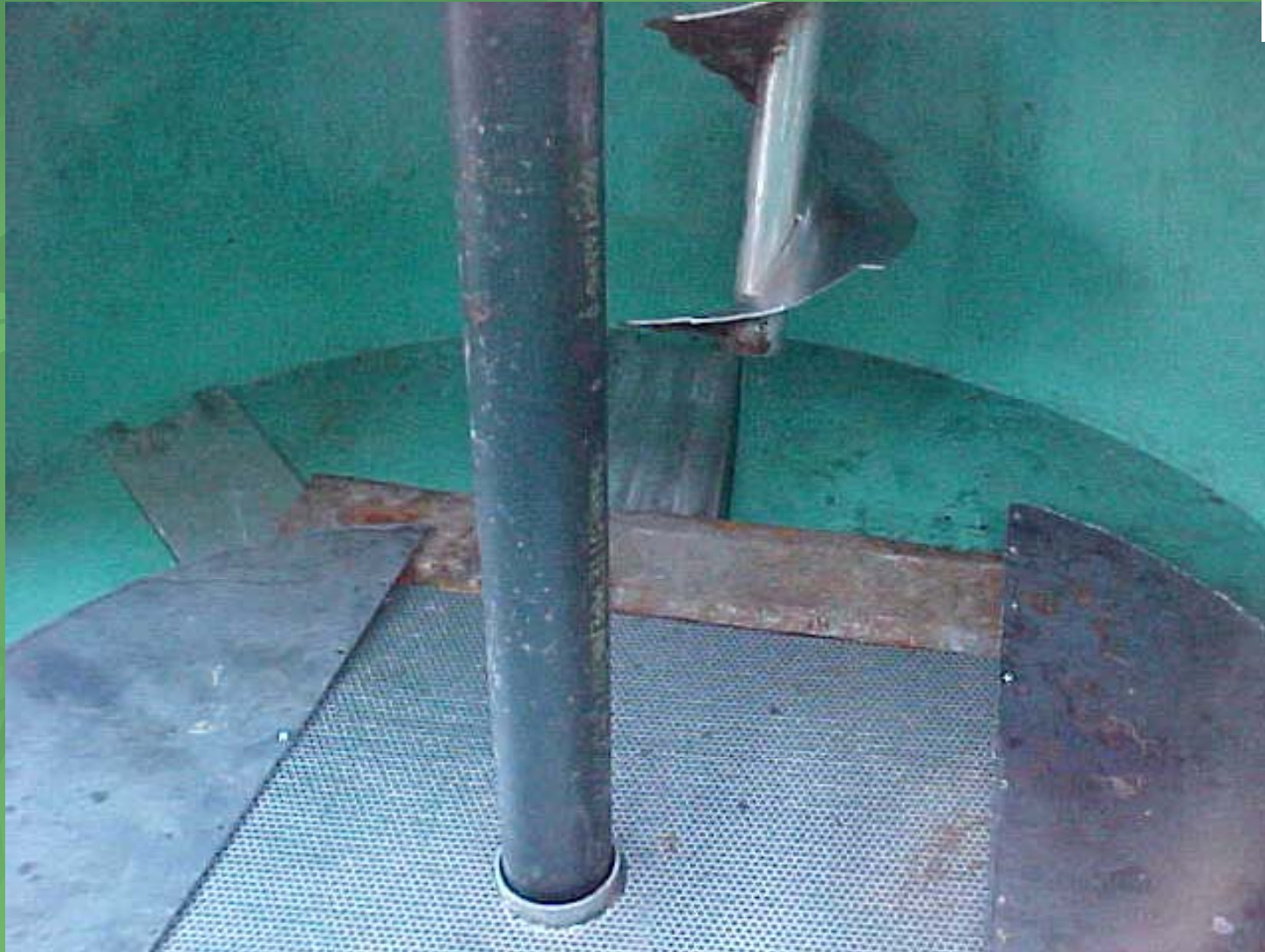
Heavy Metal Plates placed over warped areas and attached to filter grate
